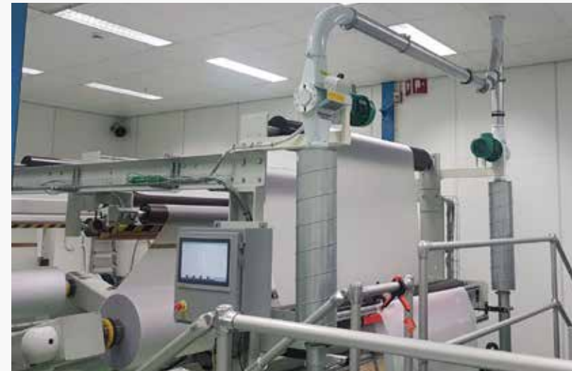
Winding and slitting machine in the clean room. Here you see the extraction points with flexible steel pipe and a MultiCutter per extraction string. Both pipes come together in one main pipe which will convey the shredded material to the waste bin.
