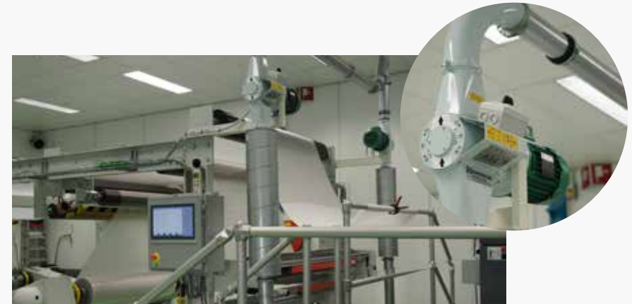
Pick-up points with two MultiCutters going into one main pipe
