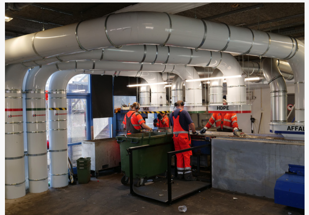
Before installation of the new pneumatic solution operators manually moved the sorted waste into collection containers.
