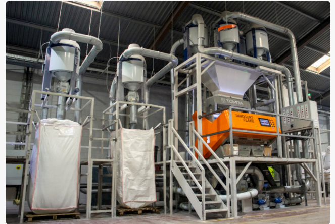
Final and reject material are discharged into big bags automatically.
