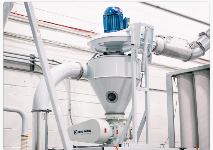
The Polyvac receives dedusted regrind from the AirWash and discharges it into Super Sack bulk bags for shipment.
