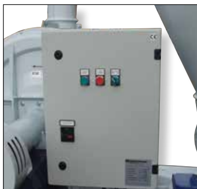
Control cabinet for automatic start/stop of the motor
