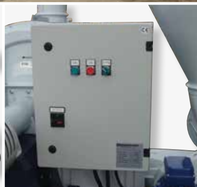
Control cabinet for automatic starting/stopping the motor.
